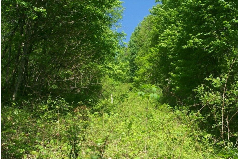
Figure 1. A 50 foot wide pipeline ROW overgrown to width of 30 feet.
