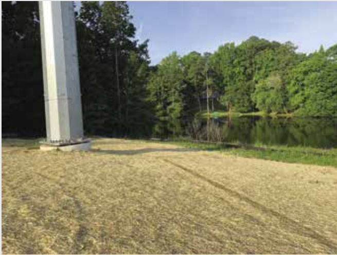
▲ Work pad stabilized with seed and straw after construction was completed. Photo courtesy of ECI.
